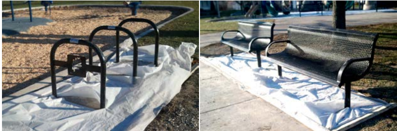
Concrete cures after new bike docking station and benches are installed in Johnsons Park.
