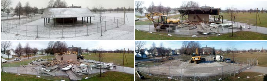
Preparation for next year's complete park renovation began with removal of the outdated pavilion.
